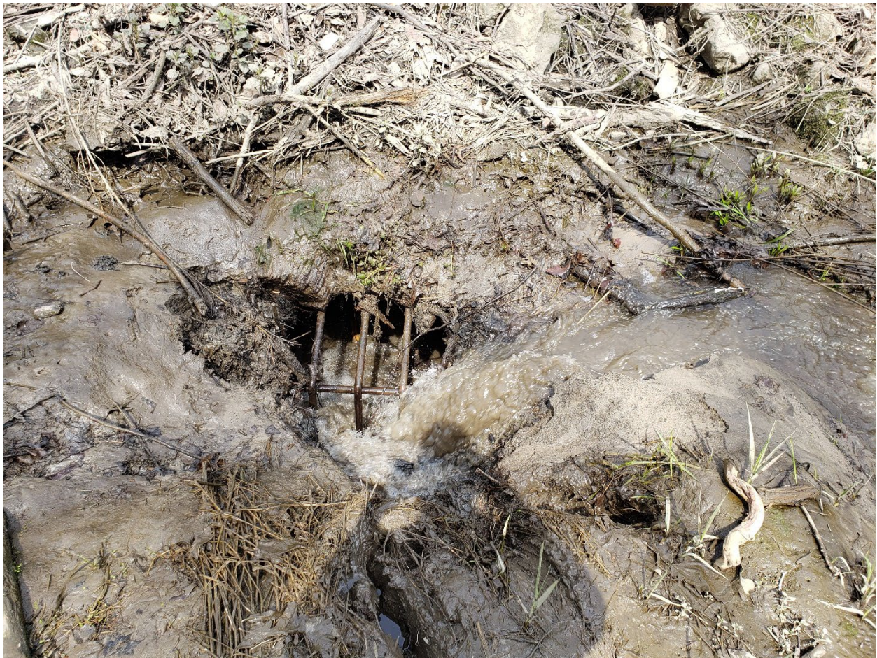
Figure 2-5 Accumulated sediment at the storm sewer pipe inlet on the west side of Kerber Blvd (photo taken by RPBCWD, May 04, 2022)
