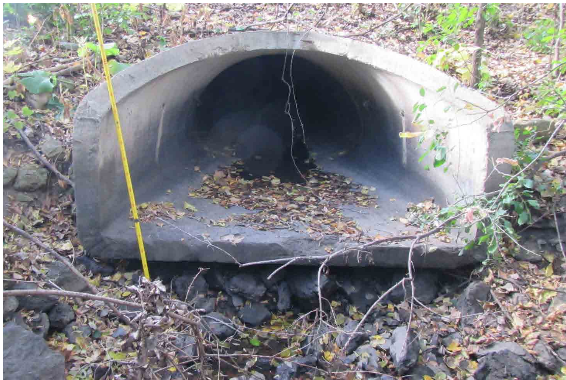
Perched stormwater outlet
