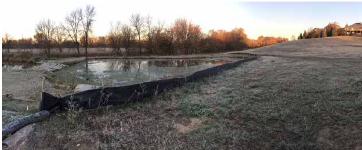
Figure 1. Fawn Hill constructed infiltration basin with standing water at the outlet elevation 7 days after precipitation event (October 22, 2018)
