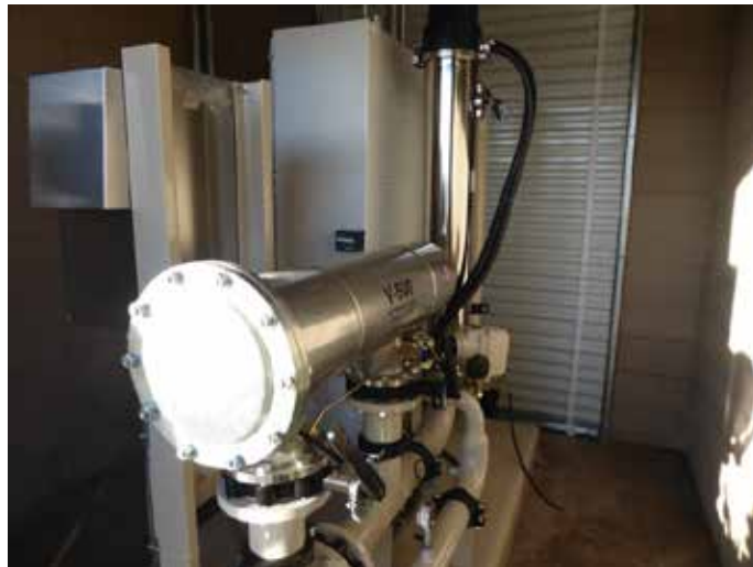
Photo: Treatment System – Automatic Filtration and UV Treatment System (by Water Tronics). 10/31/2018
